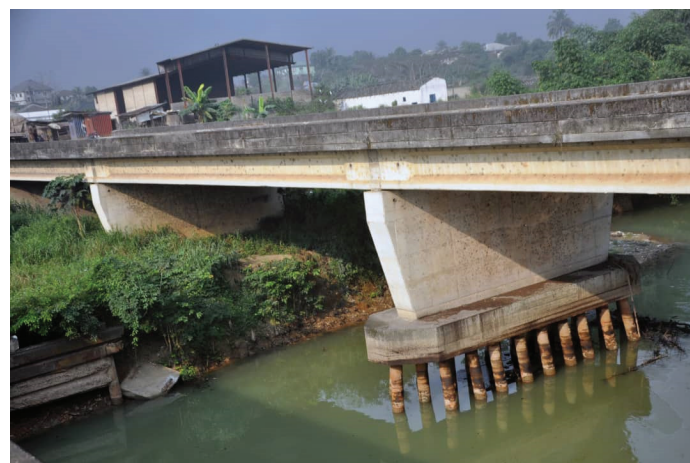
Figure 1: Bridge scouring due to sand mining at Imo river in Rivers State, Nigeria, January 2021
